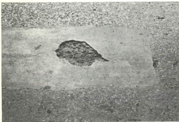
Figure 19. Continuing deterioration in and around a patched area on a bridge deck.
