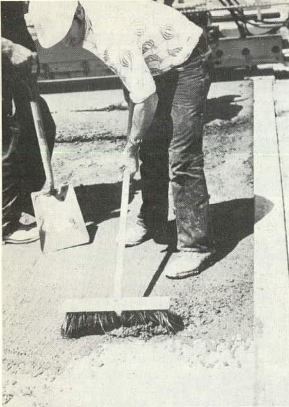
Figure 12. Application of a mortar bonding grout to a dry deck. The rate of application is controlled to prevent premature drying of the grout.
