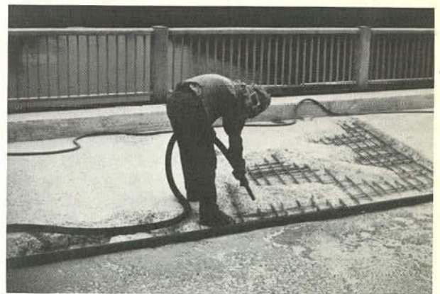
Figure 11. Sandblasting of an existing deck surface prior to application of a concrete overlay. The reinforcing steel must be thoroughly cleaned.
