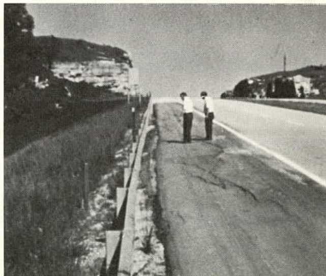
Figure 2. Visual indication of embankment failure.
