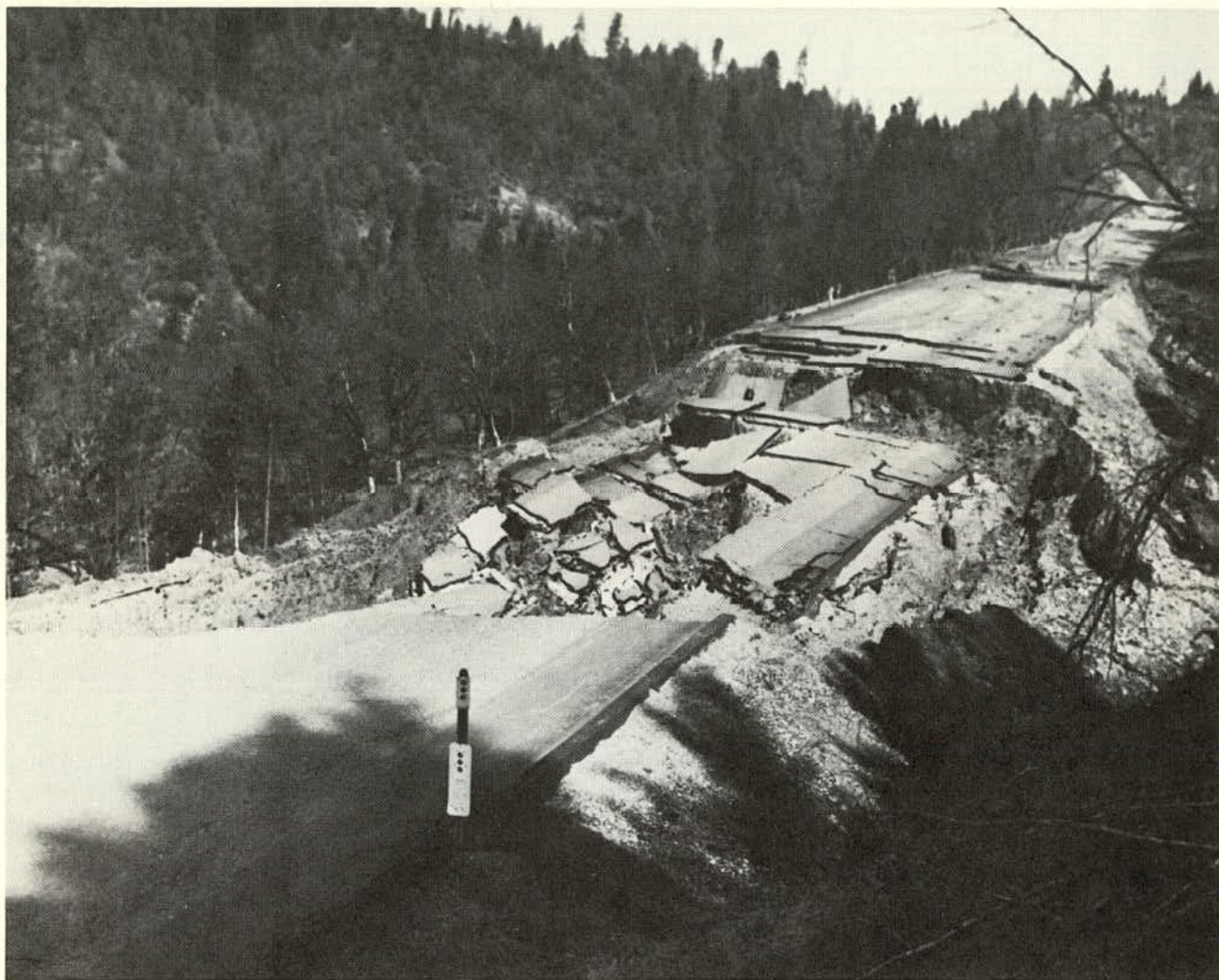
Figure 1. Massive slide failure.
