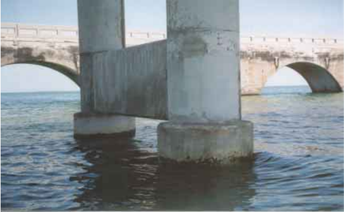
Figure D-16: Photograph of a typical bent of the Seven Mile Bridge.
