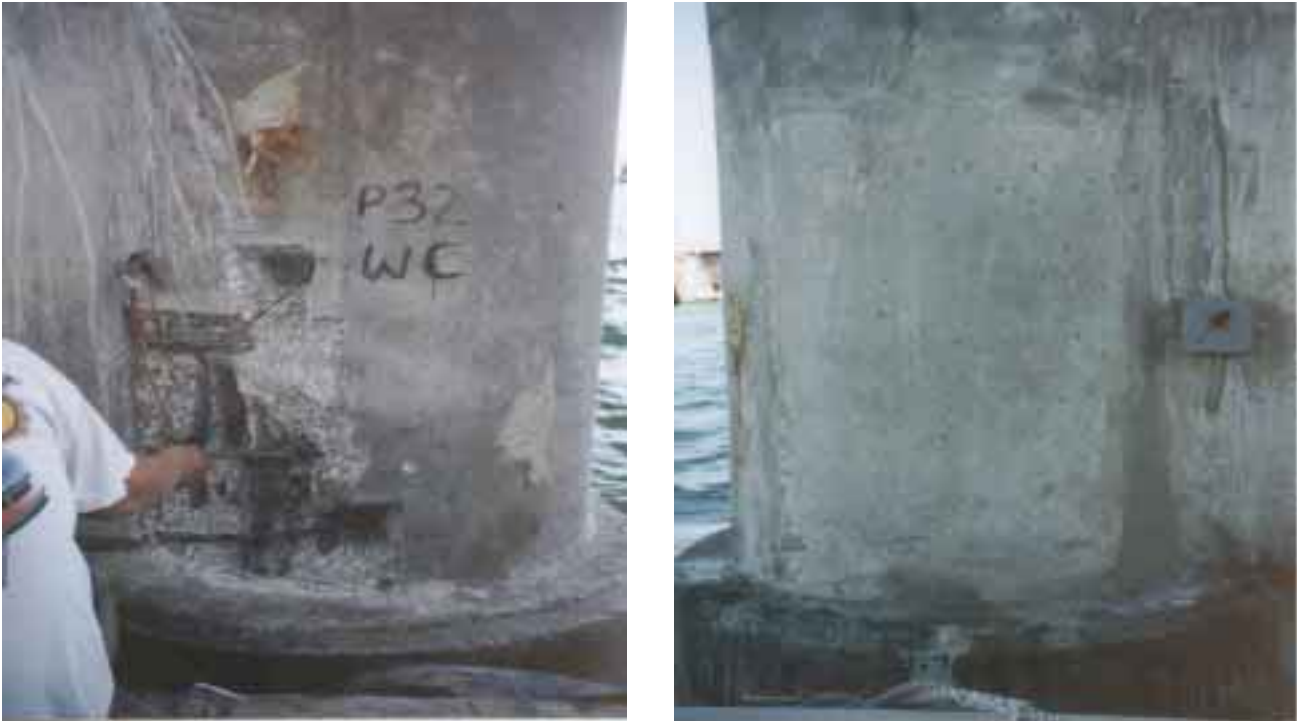
Figure D-17: Photographs showing installation of the probes and junction box for data collection.
