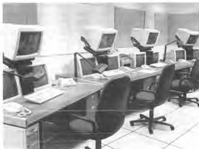
FIGURE 14 TTC Control room consoles (Toronto).
