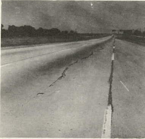
Figure 1. Longitudinal crack in CRCP.
