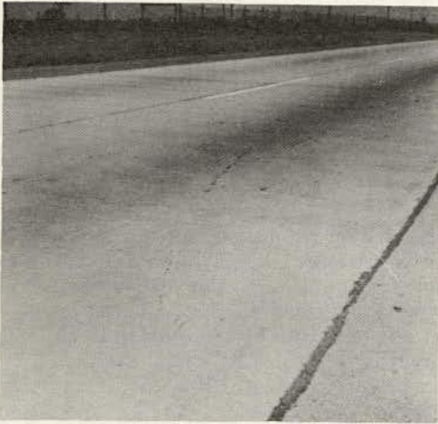
Figure 3. Longitudinal cracking with no spalling.
