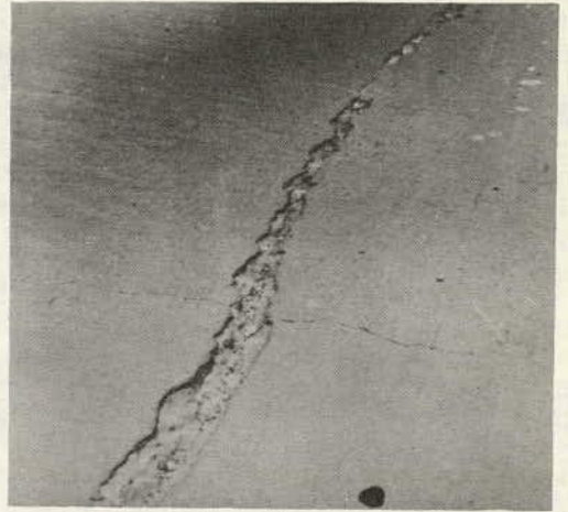
Figure 2. Close-up view of longitudinal crack.
