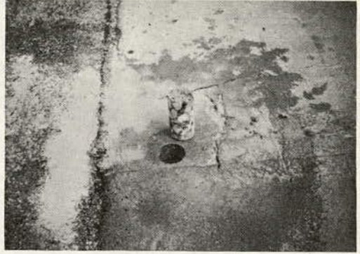
Figure 1. Areas of distress adjacent to a construction joint in CRCP (core upside down to show honeycombing).
