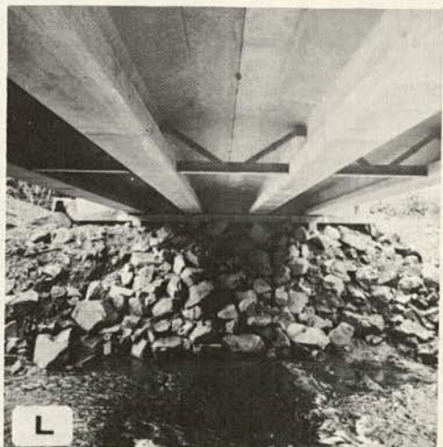
L Steel diaphragm bracing bolted to embedded steel plates to provide shear transverse between neighboring beams
