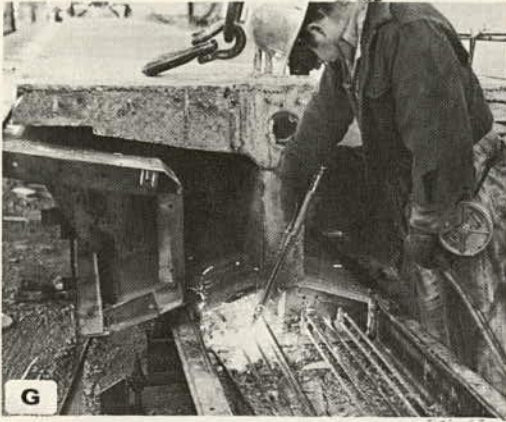
G Beam prestressed and removed from stressing bed; tension released on hydraulic rams; strands then cut with torch
