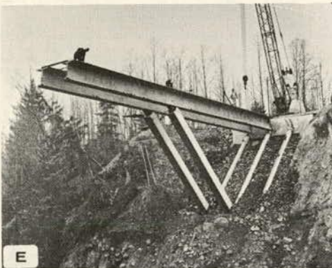
Bulb-T beams erected on pin-connected struts that are prestressed and first connected to footing
