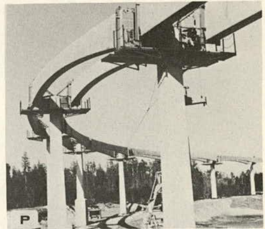
Cable ducts coupled by sleeves and gap between girders filled with cast-in-place concrete (6 girders connected into continuous spans)
