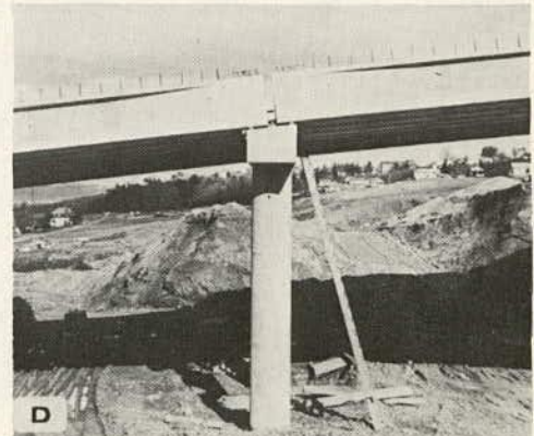
Prestressed beams on 4 x 4 in. wood blocks; space under beam ends filled with concrete for bearing
