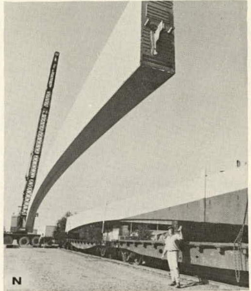
Curved girders stressed initially by post-tensioning at factory to compensate for dead-load bending (ducts for field post-tension cables project from girder end)
