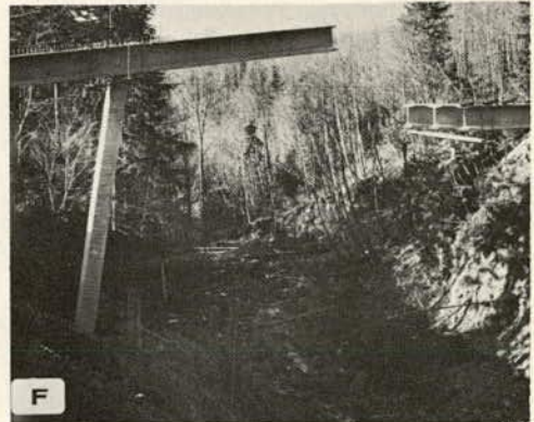
Vertically braced beam pin-connected to top hinge, walked out over canyon, and secured to abutment
