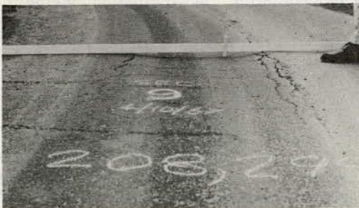
Figure 20. Further crack development and permanent deformation.
