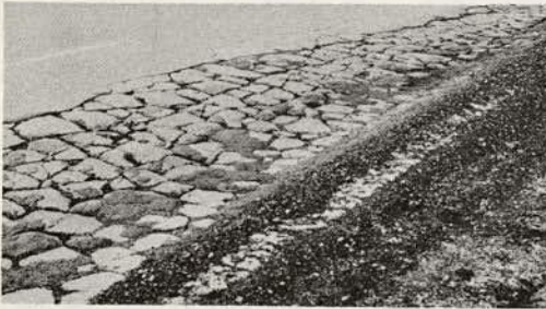
Figure 3. Complete alligator cracking prior to repair.
