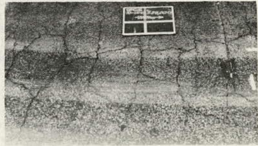
Figure 21. Ultimate form of alligator cracking covering entire trafficked area.
