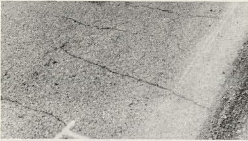
Figure 1. Initial transverse cracks in outer wheelpath of Brampton test road.
