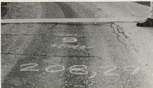
Figure 20. Further crack development and permanent deformation.
