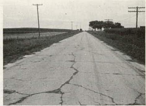
Figure 13. Crack pattern on Greene County project.
