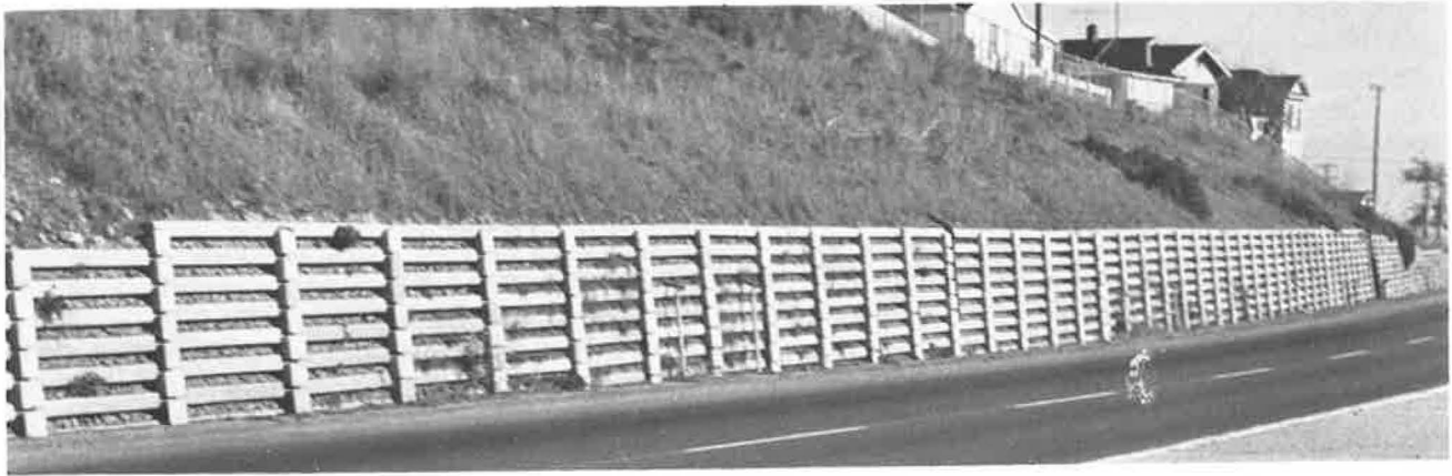
Figure 8.28. Concrete crib wall and gravel backfill installed to prevent movement in Arcata, California (8.24).
