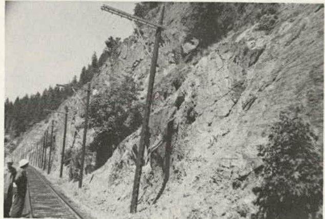
Figure 9.58. Standard type of railway electric warning fence with wires strung between upright poles and horizontal members that are cantilevered out from top of poles along Canadian National Railway line in Fraser Canyon, British Columbia.
