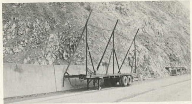
Figure 9.48. Special mobile catch fence mounted on flat deck to protect motorists from rock falls during excavation work and scaling in extremely steep terrain.
