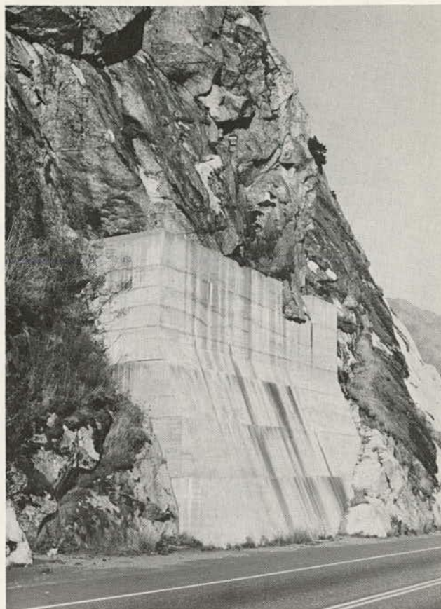
Figure 9.25. Cast-in-place reinforced concrete buttress approximately 15 m (50 ft) high providing stabilization protection of large overhanging slope.
