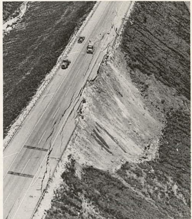
Figure 1.1. Damage to embankment on I-75 in Campbell County, Tennessee, from a landslide that occurred April 1972.
