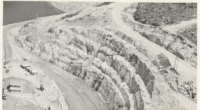
Figure 9.16. Use of multiple benches and controlled blasting techniques at Mica Dam, British Columbia, to maintain rock slope in soundest possible condition and to prevent rock falls.
