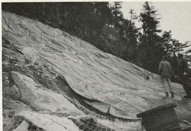
Figure 9.21. Temporary cover of polyethylene sandwiched between two layers of mesh to prevent precipitation infiltration into slope at Hell's Gate Bluffs, British Columbia.
