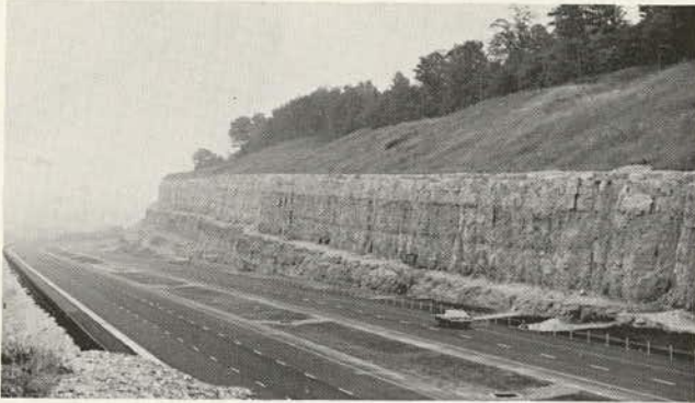
Figure 9.14. Benches that follow stratigraphy in Niagara Escarpment sedimentary rocks on Highway 403 near Hamilton, Ontario. Design also includes overburden being stripped back 3 m (10 ft) from top of rock and light fence barrier on edge of highway.
