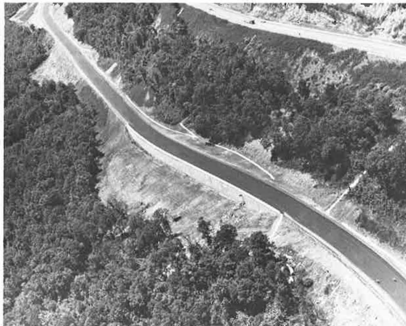
Figure 8.27. Aerial view of final correction to fill failure using reinforced earth, I-40 near Rockwood, Tennessee (8.26).
