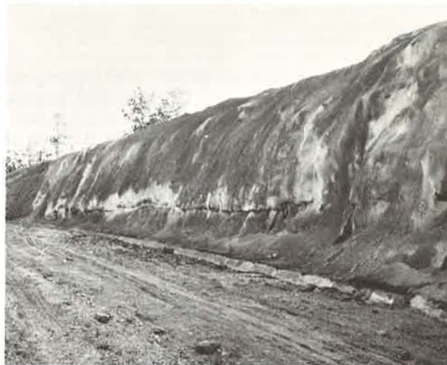
Figure 8.5. Slope protected by pneumatically applied mortar.
