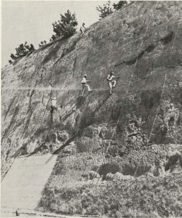
Figure 9.43. Anchored double-twist, hexagonal wire mesh being fastened on a high rock face to prevent rock falls onto highway.
