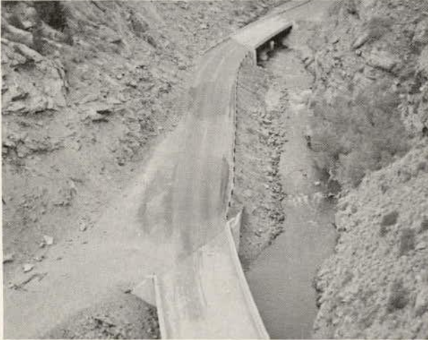
Figure 3.37. Early signs of impending debris slide along Clear Creek, Colorado (3.10). Displacement of fence, bulging of pavement, and distress in bridge abutment (Figure 3.38) all give early indications of movement at toe of incipient slide. In several places, now covered by patching, centerline stripe was offset along cracks.
