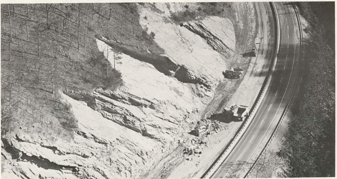
Figure 4.8. Slide in sandstone overlying shale in Tennessee.
