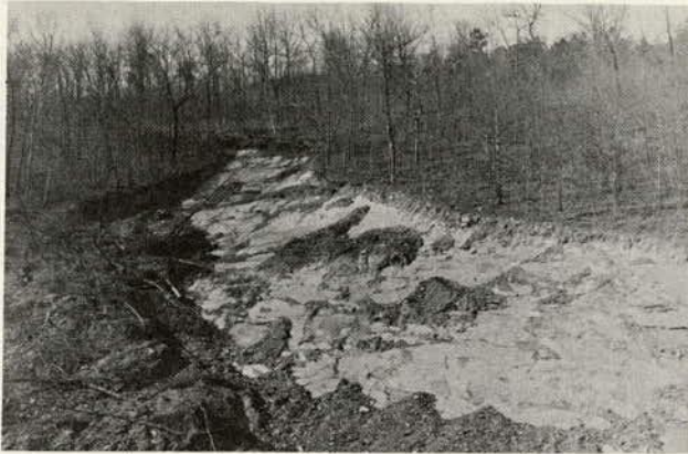
Figure 2.11. Thin layer of residual debris that slid on inclined strata of metasilstone along I-40 in Cocke County, Tennessee.
