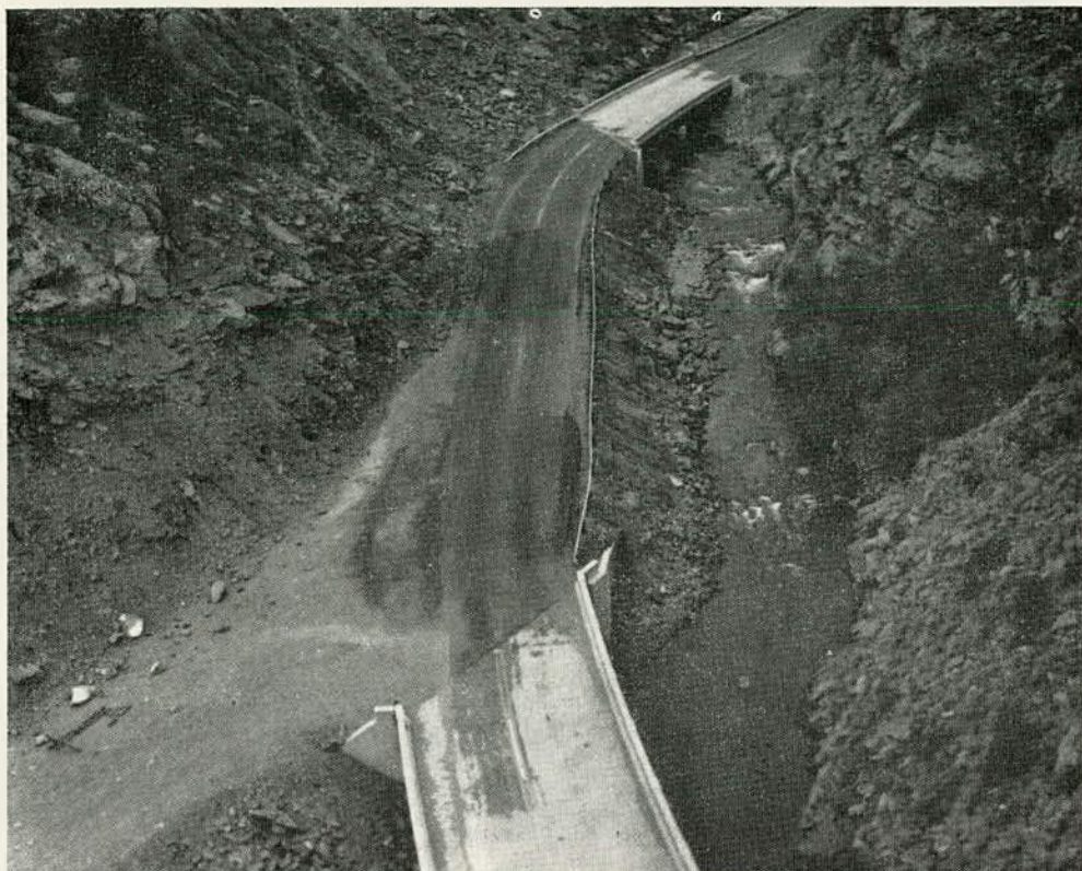
Figure 34. Early signs of impending debris slide, highway along Clear Creek, Colo. Displacement of fence, upbulge of pavement, and distress in bridge abutments (see also Figure 35) all gave early indications of movement at the toe of an incipient slide. In several places, now covered by patching, the centerline stripe was offset along cracks. (Photograph by D. J. Varnes, U. S. Geological Survey)
