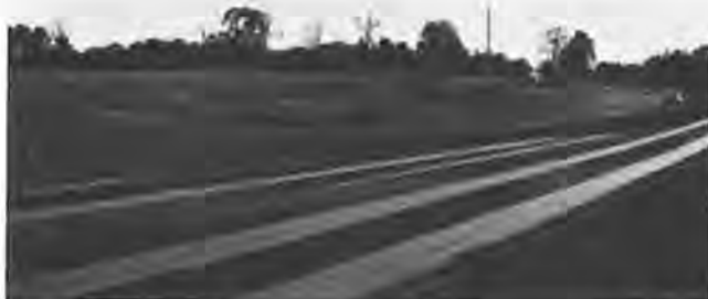
FIGURE 3 Extreme variation in friction (skid number of the advance pavement is 70, and skid number where the wheel paths have flushed is less than 10).
