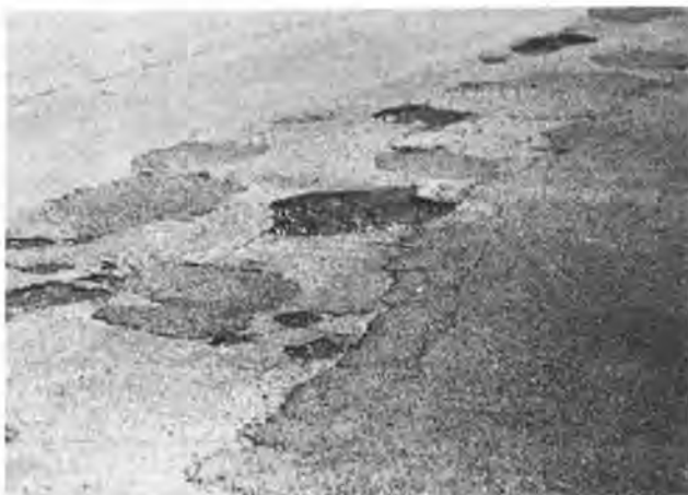
FIGURE 1 Potholes and bumps in combination.
