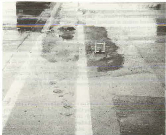
FIGURE 3 AC patching of slab deterioration.
