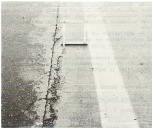
FIGURE 2 Spalling of longitudinal joint between the PCC slab and the asphalt concrete.
