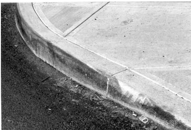
Figure A-45. Evidence of automobiles hitting curb on bulb.
