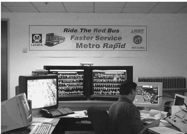
Photo 7-E. Central control room, Metro Rapid, Los Angeles.
