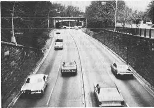
Illustration 2.1 Lane width and lateral clearance problems are evident on this old section of parkway.
