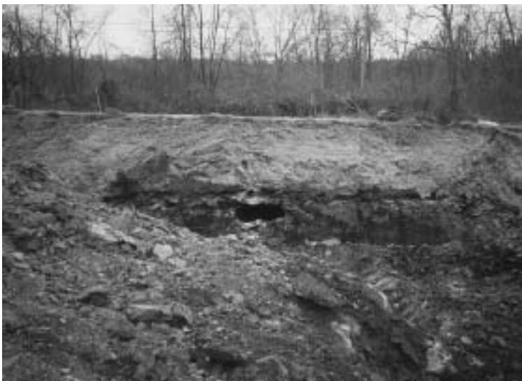
Exposed mine void beneath State Route 32.
