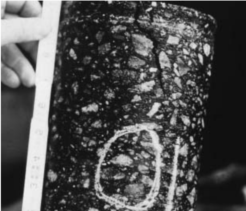
Core sample from I-287, showing top-down cracking.
