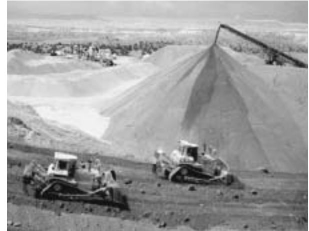
Alternate aggregate source material, suggested by value engineering program, played important role in construction on NM 44.
