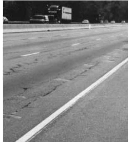
In 1993, after 26 years of service, New Jersey I-287 (above) appeared to be in terminal condition.
