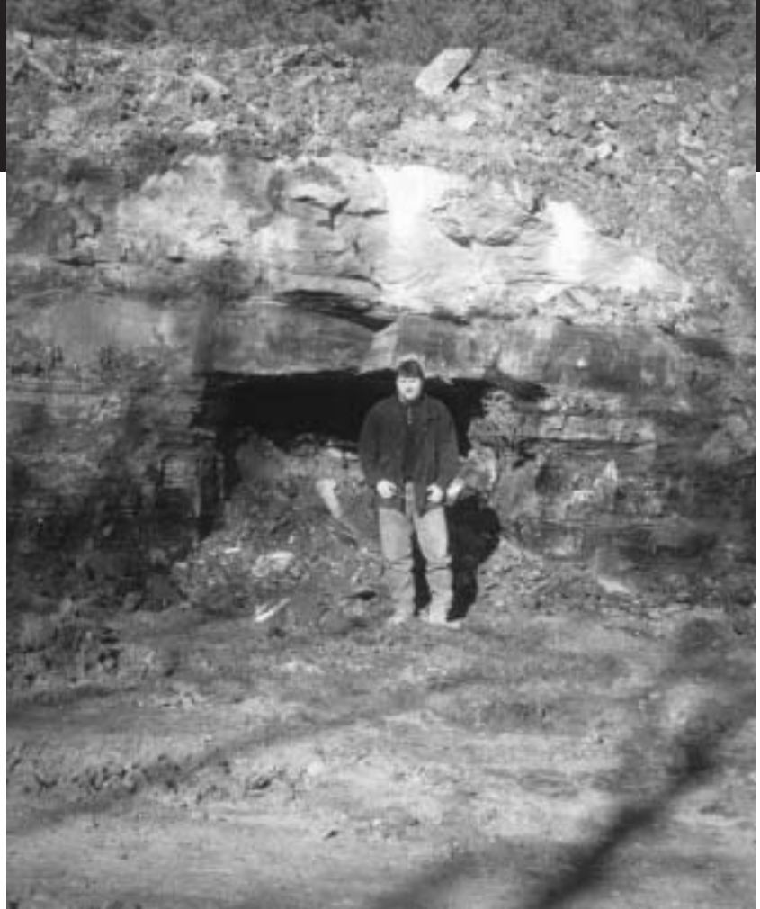
Ohio DOT employee in front of four-foot-high void discovered underneath eastbound lanes of State Route 32.
