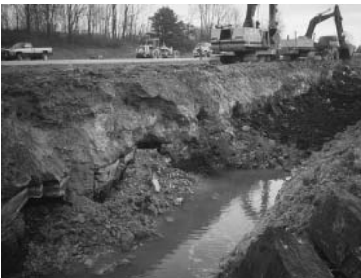
Eighteen-foot trench after excavation of the overburden and mined coal seam. Note the exposed mine openings.
