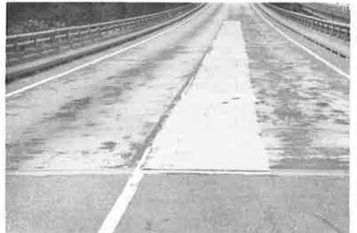
Figure 6. Coal-tar epoxy on deck of northbound Meherrin River bridge.
