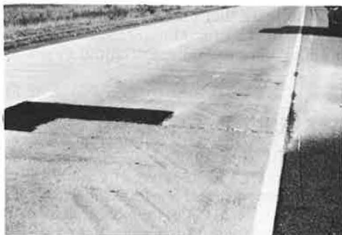
Figure 8. CRCP failure due to poor consolidation.
