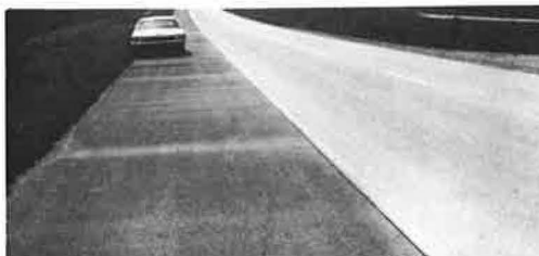
Figure 10. CRCP edge pumping due to poor drainage of shoulder material.
