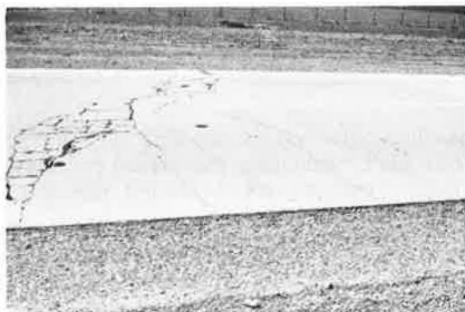
Figure 1. Fragmental distress at lapped splices on US-82 in Leflore County.
