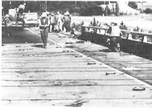
Figure 6. Anodes on concrete surface.
