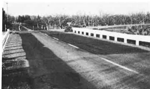
Figure 5. Sutter County test bridge: 30 percent TKPP has been applied to right side of bridge; note frost on left side.
