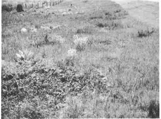
Figure 1. Unsprayed section of I-69 near the Indiana-Michigan border. Tall weeds and grass have smothered out the turf leaving patches of bare soil subject to erosion. Photographed June 2, 1973.
