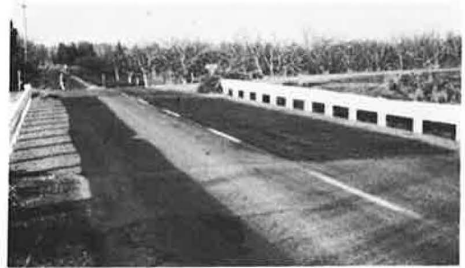
Figure 5. Sutter County test bridge: 30 percent TKPP has been applied to right side of bridge; note frost on left side.
