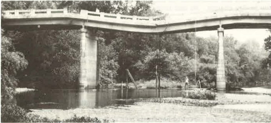
Figure 5. Bridge B at failure.
