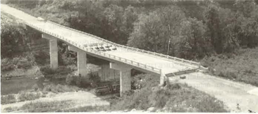
Figure 4. Bridge A at failure.
