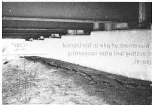
Figure 4. Breakup of slope protection beneath bridge deck.
