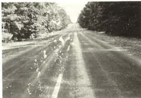
Figure 6. Binder demand may vary across pavement and transverse adjustment of spray bar output may be required.
