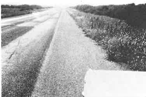
Figure 4. Lack of uniformity of surface to be sealed.
