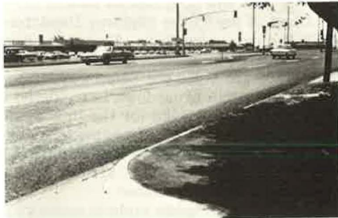
Figure 5. Shaded areas of seals using emulsions develop bond more slowly than exposed areas.
