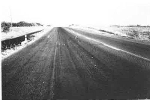
Figure 1. Flushing seal coat caused by unexpected truck traffic.
