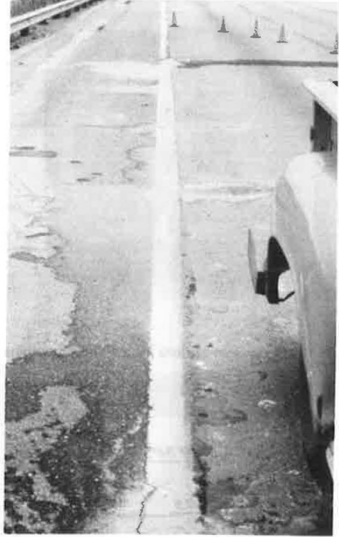
Figure 22. Water in depression between pavement and shoulder.
