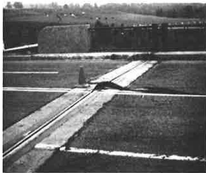
Figure 3. Installing strip seal element in one piece, a lane at a time, for 100 percent leakproofing.
