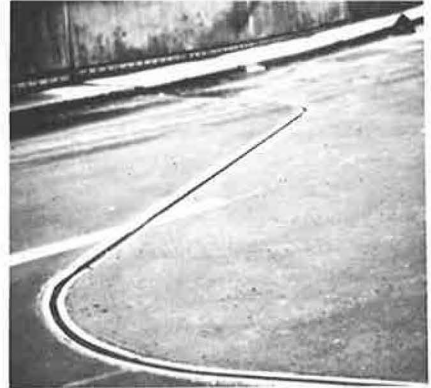
Figure 21. Unusually curved joint in Cologne-Bonn Airport upper departure level structure sealed with single-tube system.
