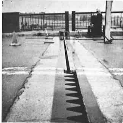
Figure 2. Seam-welded steel extrusion replacing old finger joint.
