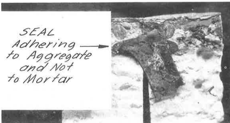
Figure 16. Seal failing in adhesion in section 4.
