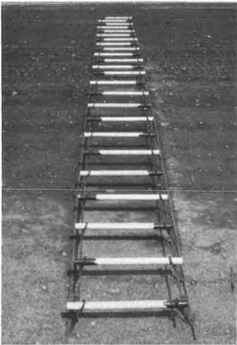
Figure 6. Bare dowel ends painted with red lead.
