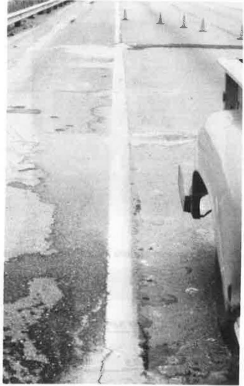
Figure 22. Water in depression between pavement and shoulder.
