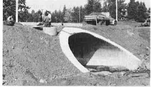
Figure 2. End view of completed structure with test load truck, readout station, and relief slab.
