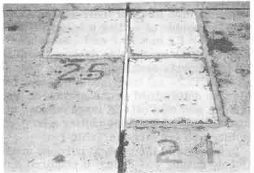
Figure 9. Patched area requiring more than one slab.
