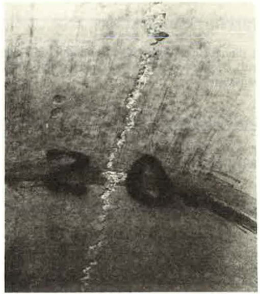
Figure 4. Cracks in conduit at crown.
