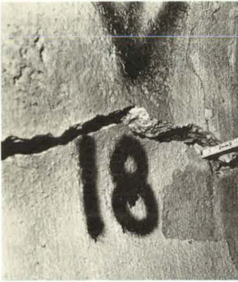
Figure 3. Cracks in conduit at spring line.
