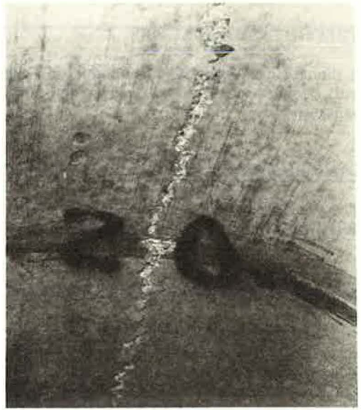
Figure 4. Cracks in conduit at crown.
