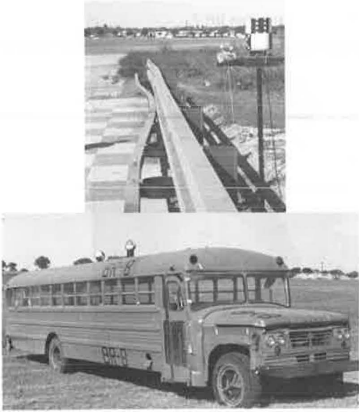
Figure 11. Condition of vehicle and collapsing-ring bridge rail after impact in test BR-8.
