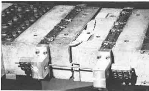
Figure 12. Damaged expansion joint.
