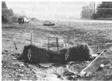
Figure 2. Improperly constructed and maintained filter barrier.
