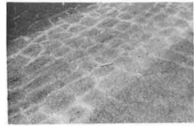
Figure 5. Crack pattern under asphalt-rubber seal.
