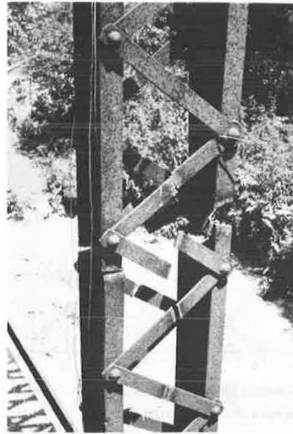
Figure 7. Damaged member after collapse.
