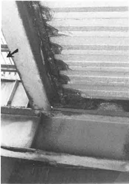
Figure 4. Corrosion of forms in vicinity of grating type of drainage feature.
