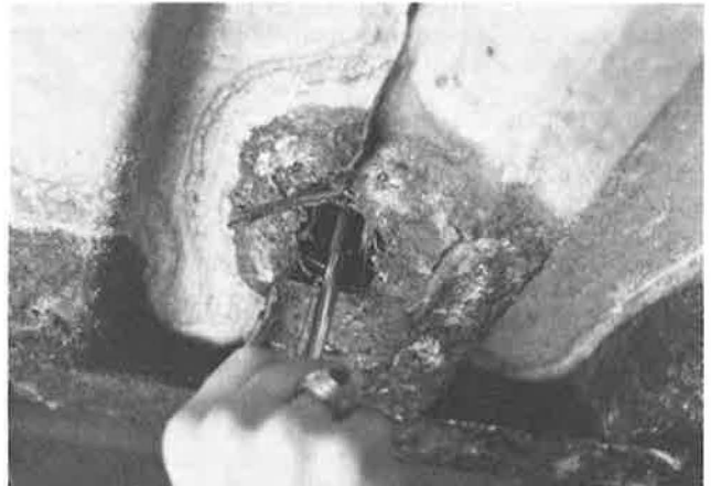
Figure 7. Corroded form and deteriorated concrete at location of foreign material in deck.
