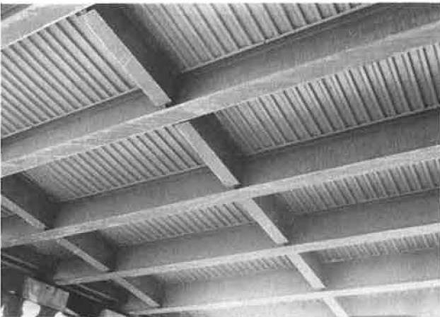
Figure 2. General condition of forms.
