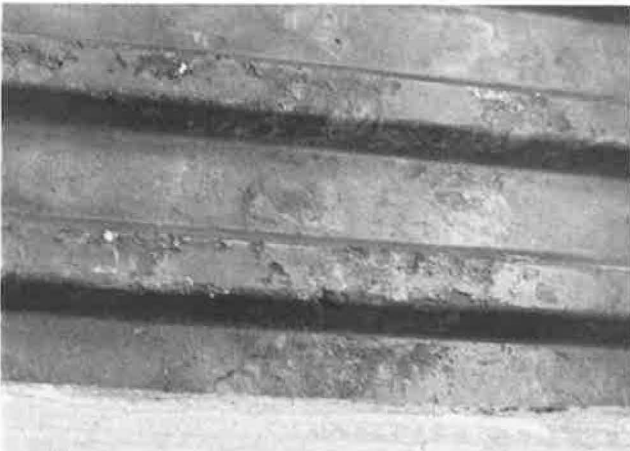
Figure 5. Condition of concrete in form removal area.
