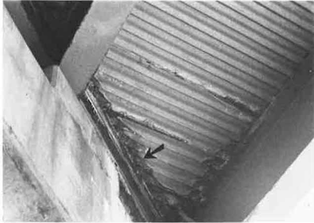
Figure 3. Corrosion of forms near span end and along fascia girder.
