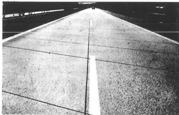
Figure 1: General view of the highway (1970) showing the grooving of 1970 with groove distances of 2,0 m.
