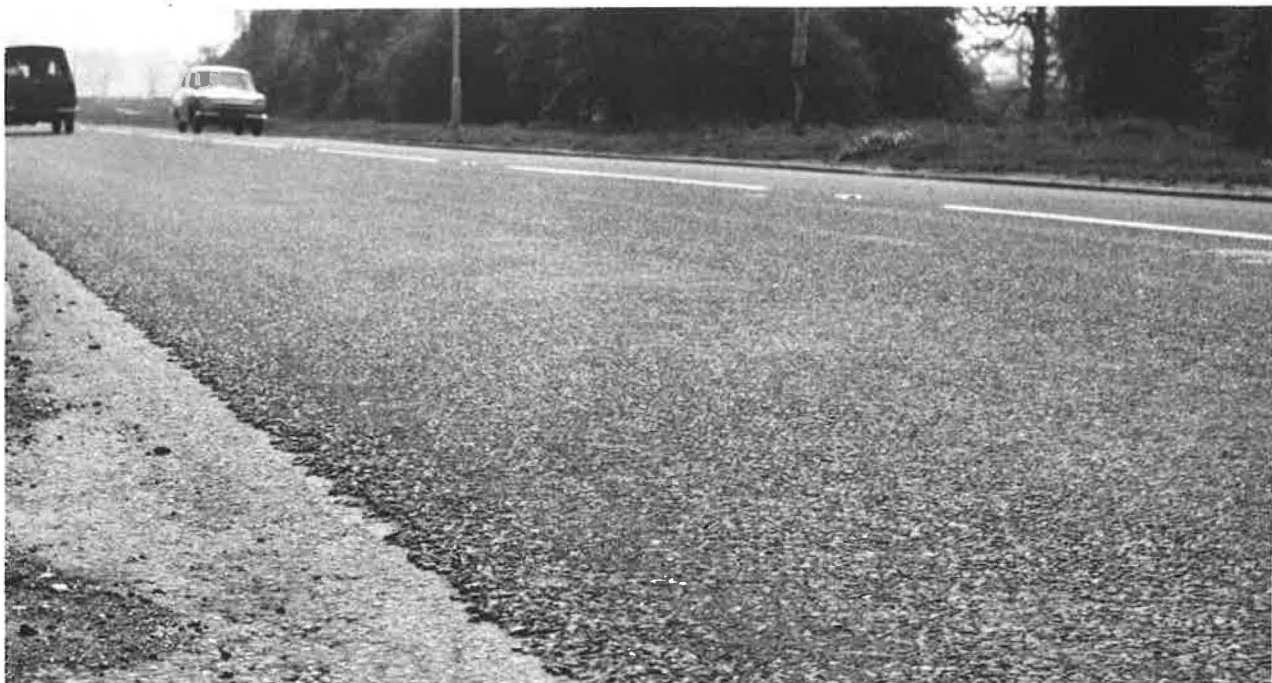
Figure 8 Example of surface dressing with high-viscosity cutback after 2 years. A41 road, Bushey, England.
