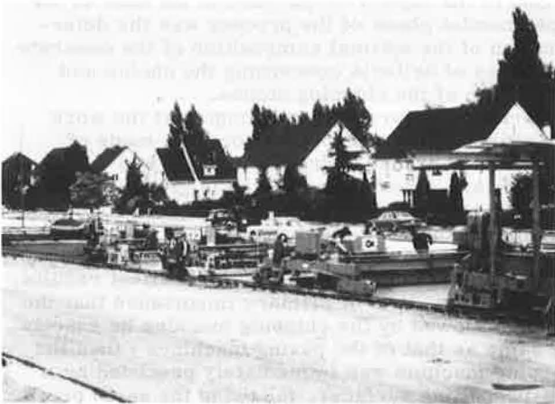
Figure 2. Paving train for the application of a pavement in chipped cement concrete. Width of work : 7.50 m (25 ft.).
