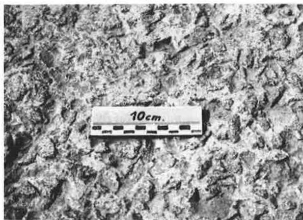
Figure 1. Aspect of chipped concrete after 21 years of traffic.
