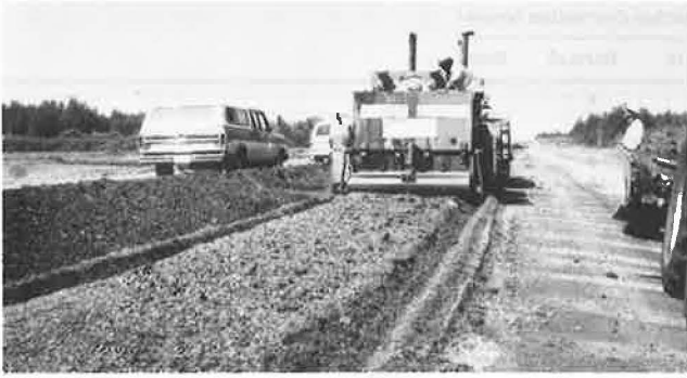
Figure 8. Pulverization by using a heavy duty Hammermill pulverizer.
