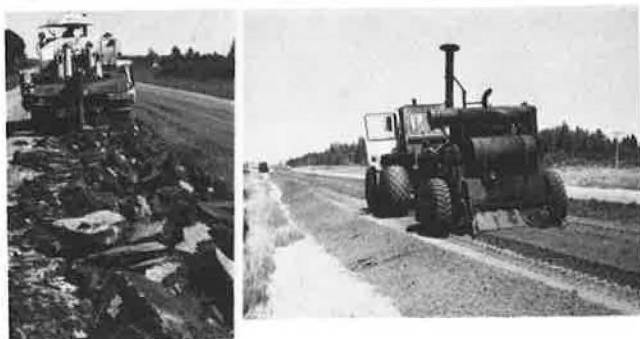
Figure 7. Pulverization by using a Hammermill pulverizer.
