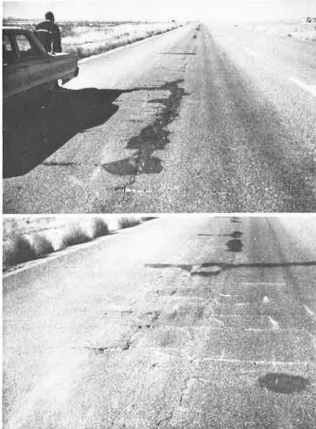
Figure 1. Typical roadway cracking on Minnetonka-East, February 1969.
