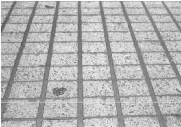
Figure 2. General surface condition of concrete-filled steel-grid bridge deck with no wearing surface after 42 years service (bridge 18).
