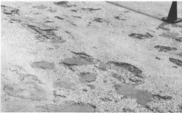
Figure 1. Deck in need of resurfacing.
