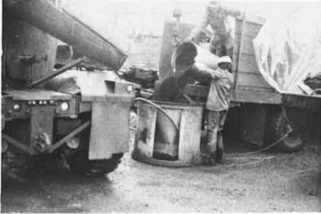
Figure 15. Wax beads being added by concrete bucket to already mixed concrete at jobsite.
