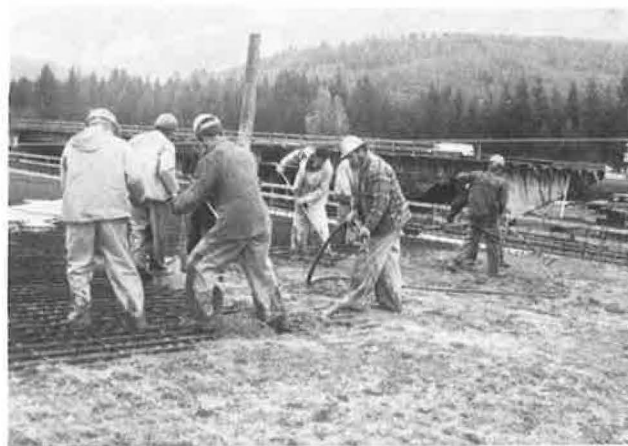
Figure 13. Lower course of conventional concrete being raked off at level of top mat of reinforcing steel after placement and consolidation by internal vibration.
