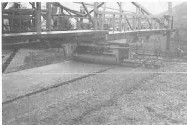
Figure 14. Bidwell finishing machine in operation with vibrating pad located between rollers and strike-off auger.
