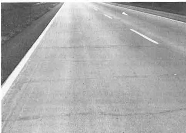
Figure 4. Heavy-burlapped texture after 6 years under traffic.
