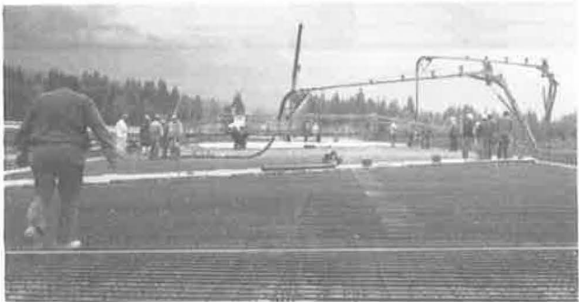
Figure 12. Bridge deck pour in operation: concrete pump in foreground placing standard class AX concrete and pump in background placing wax-bead concrete overlay.
