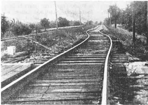
Figure 9. Thermally buckled track.
