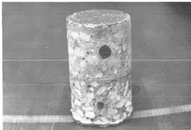
Figure 3. Core from 7 year old panel deck.
