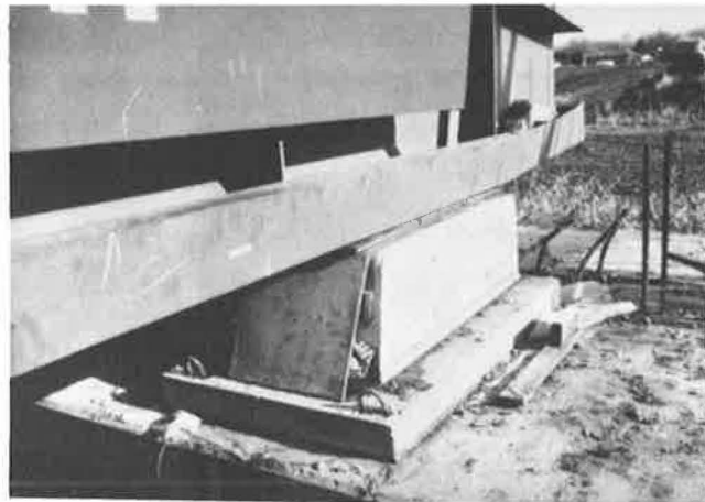
Figure 20. Teflon-faced neoprene pads on temporary sliding bearings.
